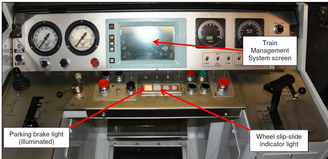
Figure 13: Tangara driver control panel
