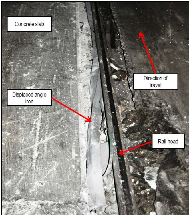
Figure 2: Concrete Slab with displaced angle iron
